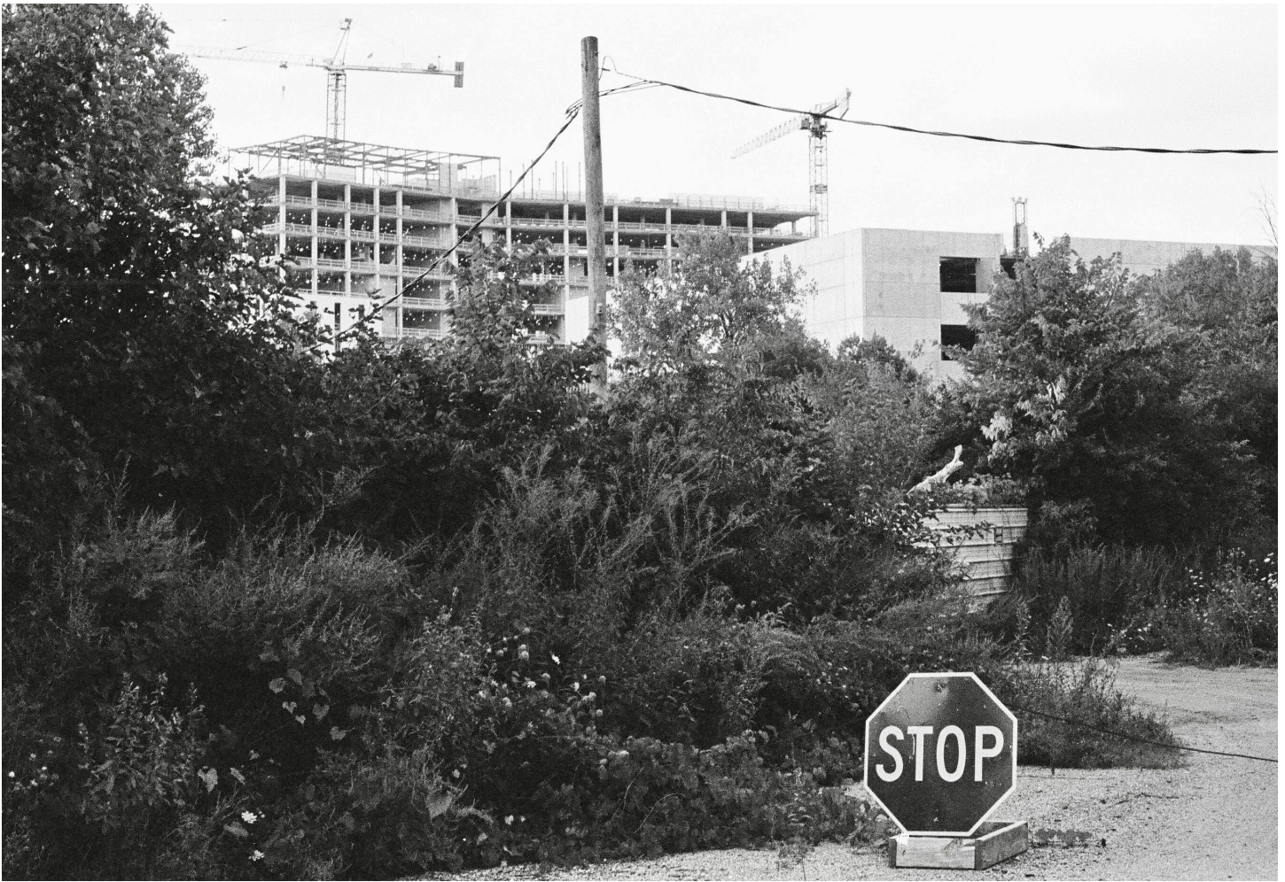
The new Marion County Community Justice Campus under construction in 2020. The campus will replace the current county jail and court facilities.
